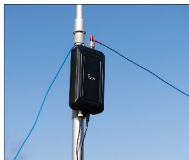
Wire antenna installation example
